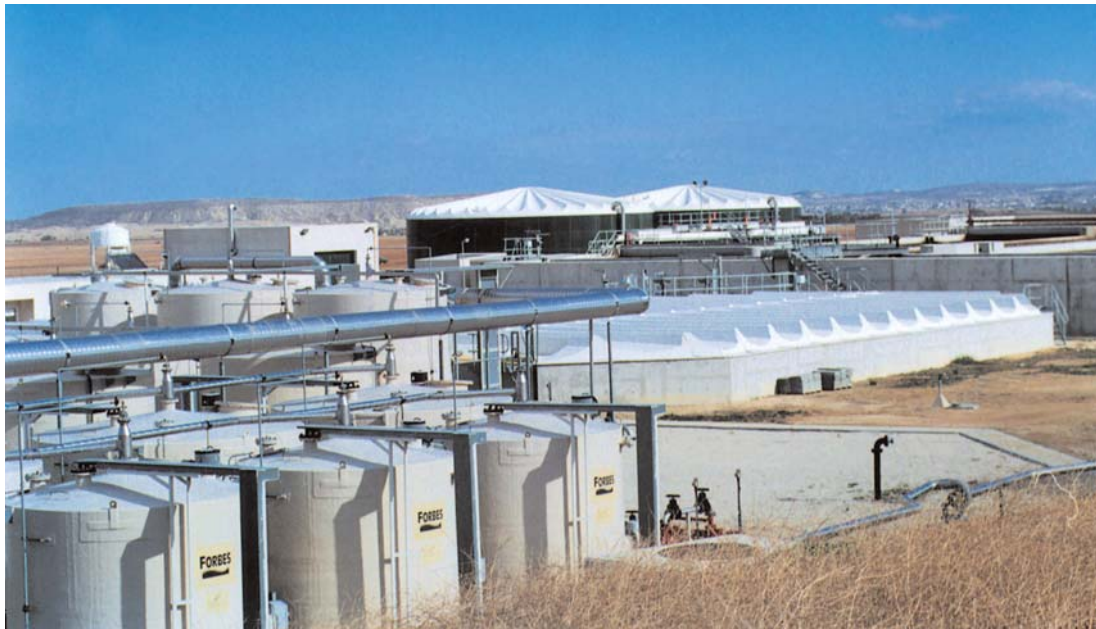
House sewage and industrial waste treatment plant at Vathia Gonia (Photo: Ministry of Agriculture, Nat. Res. & Env. Archive)
