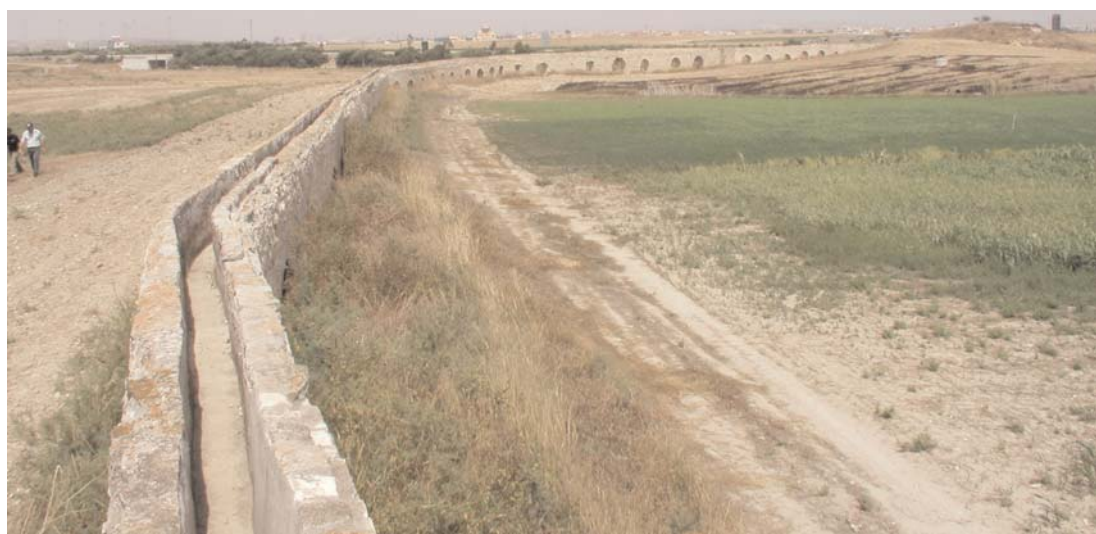
Masonry aqueduct for the water supply of the town of Larnaca (Photo: WDD Archive)
