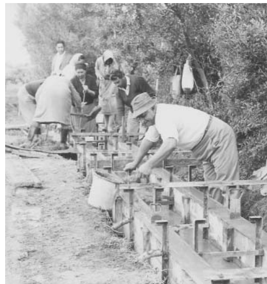
Construction of irrigation canals (Photo: Ministry of Agriculture, Nat. Res. & Env. Archive)
