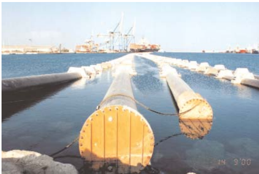
Placing pipelines in the sea during the execution of the construction works of the Larnaca desalination unit.
