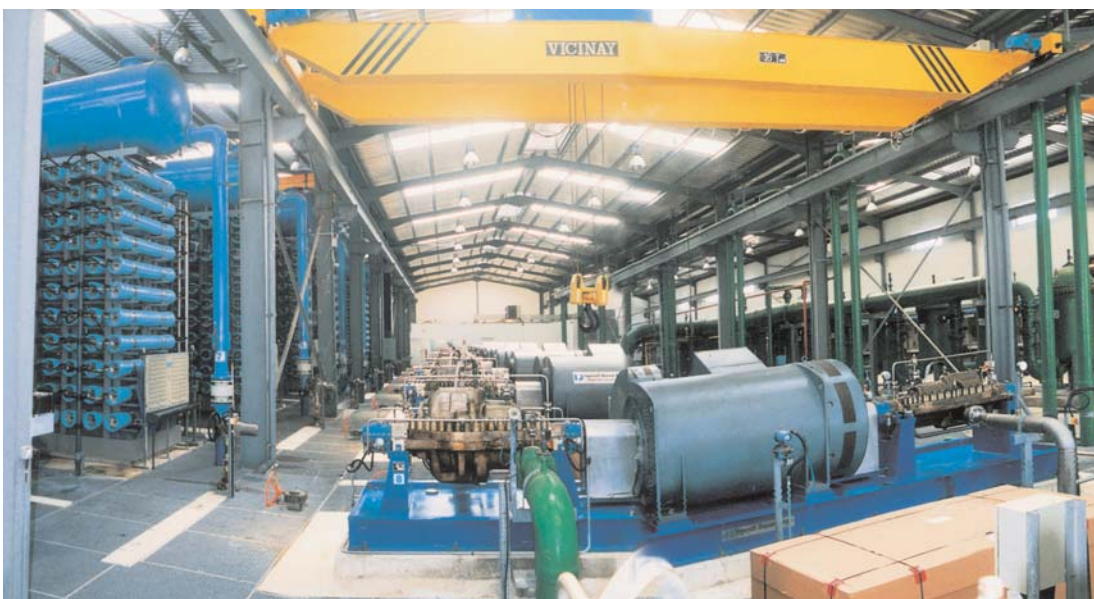
Dekelia desalination unit.
