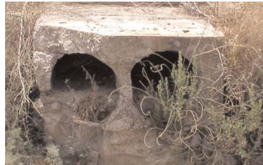
Underground masonry conveyors that conveyed water from the "laoumia" to the stone aqueducts for the water supply of the town of Larnaca (Photo: WDD Archive)
